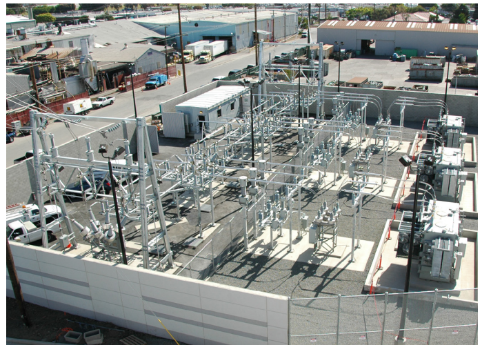
DuPont Fabros Substation Project
