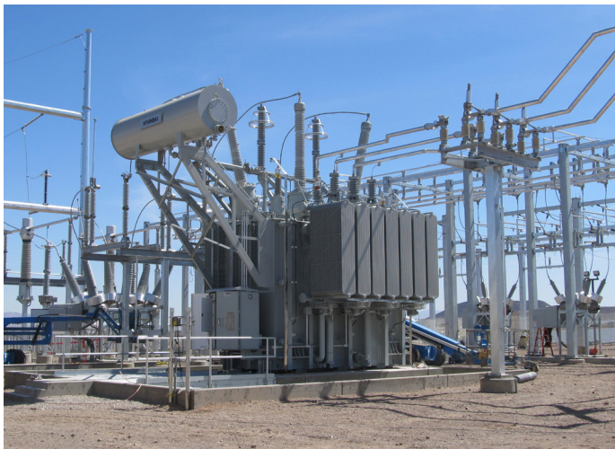
Copper Mountain Solar 2 Substation Project
