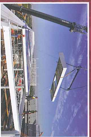
Wiring of 1,150 solar panels located across Solar Terrace on Green Roof (174kW) and three 'Energy Bridges' (210 kW)
