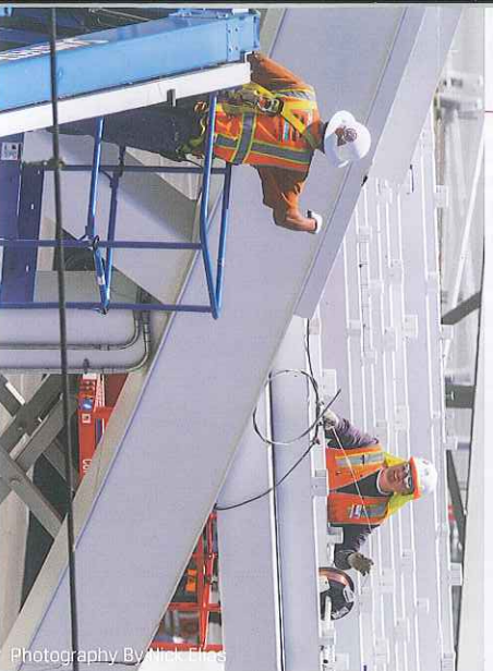
Cupertino Electric installed solar panels on three 'energy bridges' and on the green roof.
