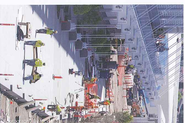
At the peak of construction Cupertino Electric employed 270 electricians and 60 technicians, all from IBEW Local 332 in San Jose.
