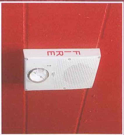
Wiring for state-of-the-art Fire Alarm System Controls, including Mass Notification Controls and Speaker/ Strobe Fire Detectors located throughout the stadium.
